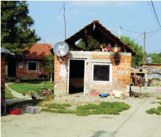
An example of sub-standard housing in a remote Roma settlement.
