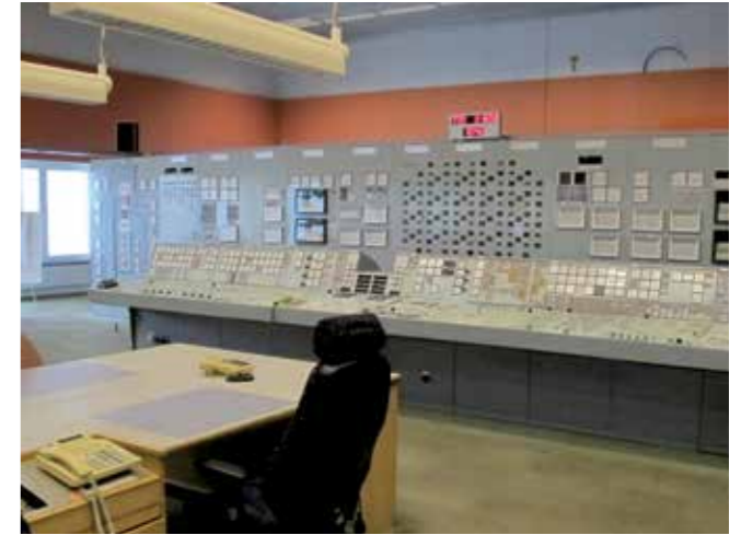
The control rooms at Barsebäck nuclear power plant today stands mostly empty and silent, awaiting the planned demolition of the plant.
