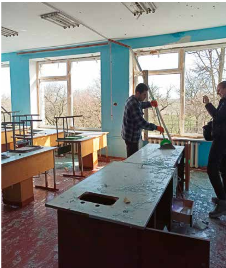
Inside destroyed secondary school in Makariv region, April, 2022.
