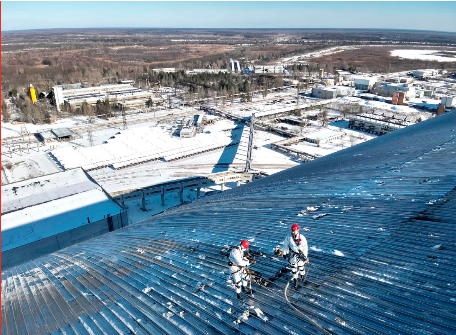
On February 14, 2025, a drone hit the Chernobyl New Safe Confinement, damaging the sarcophagus. The repair operation required workers to ascend 100 metres in extremely difficult weather conditions.
